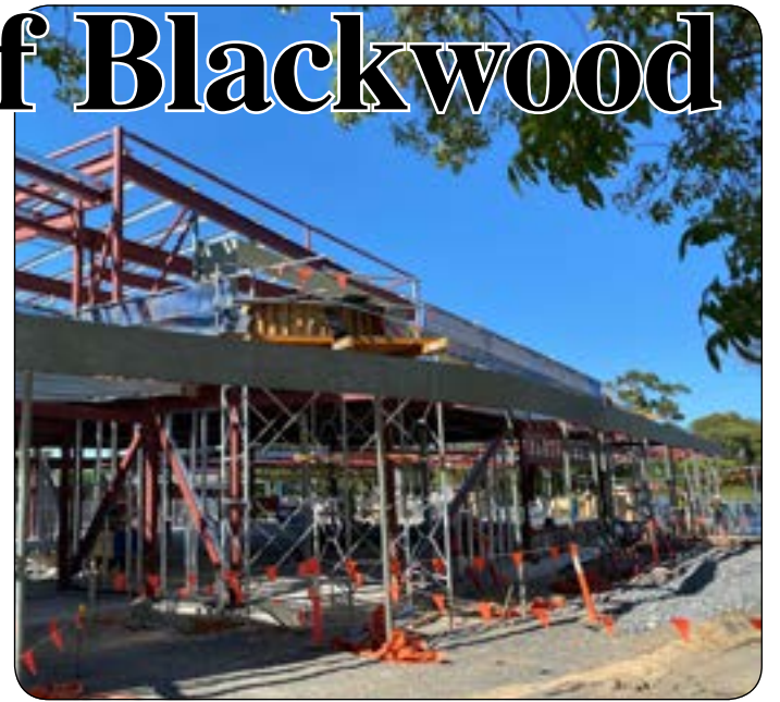
◆ Photo - The Blackwood Community Hub & Library is starting to take shape as installation of steel framework commenced during January
