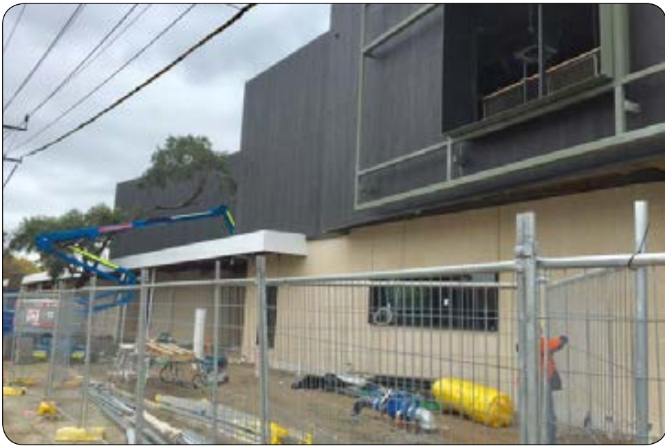
◆ Photo - Blackwood Community Hub & Library ('Tiwi Kumangka') is full steam ahead with a planned completion date in August and official opening in September
