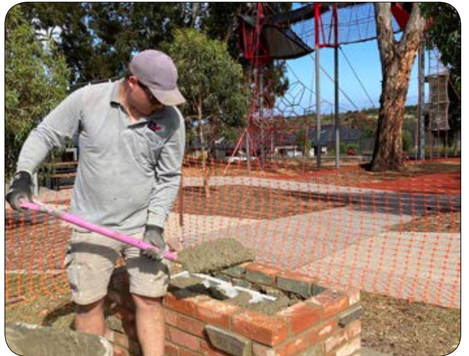
Photo - Craighburn Farm resident from Built Right Masonry Constructions preparing the base for the commemorative table near Blackwood Park Treetops playground
