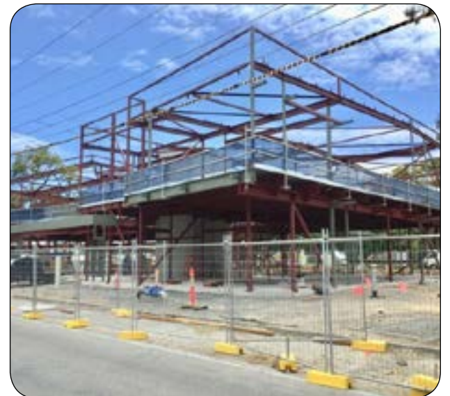
◆ Photo - Steelwork for the Blackwood Community Hub & Library being constructed in Young Street, has been completed including the structural steel to perimeter canopy and purlins. Now, the first floor services can be installed and the upper floor cement poured. It is anticipated that the Hub will be completed in July 2023.
